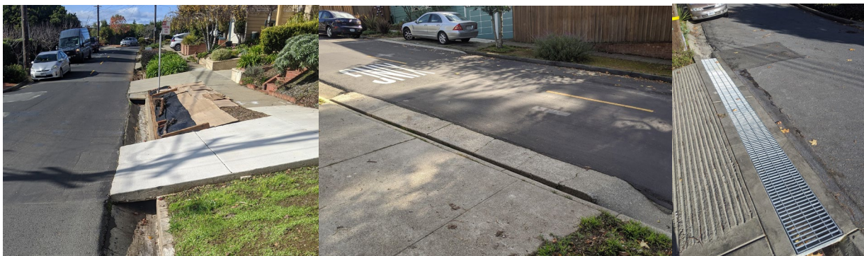
Figure 8: Three variations of driveway gutter crossings: Hard edge (left), smooth edge (center), and metal grate (right).
